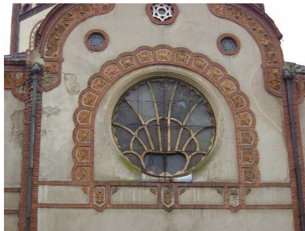
Figure 3. Detail of the north façade damaged by water (Authors photograph from 2000)
