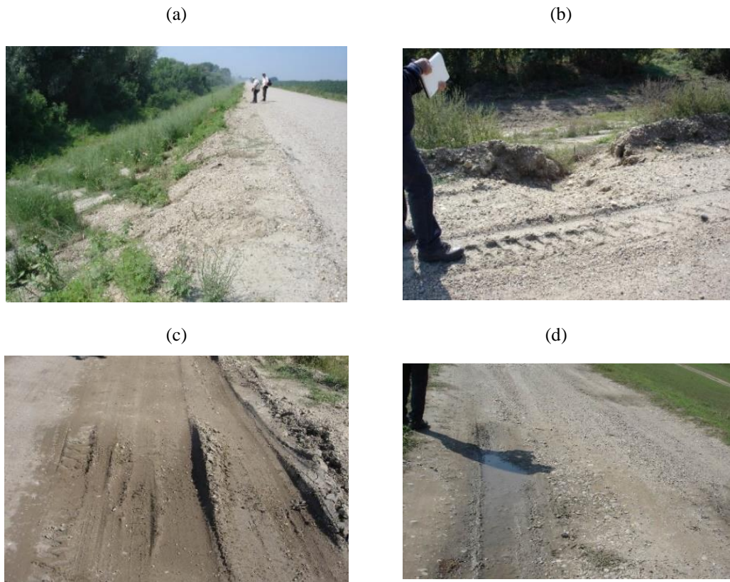
Figure 11 Registered types of deformations on the embankment: (a) Type I of deformations: overflow of the added sand-gravel material over the basic embankment; (b) Type II deformations: gutters - erosion furrows along the perimeter of the embankment crown; (c) Type III deformations: depressions on the road; (d) Type IV deformation: holes in the crown of the old embankment.
