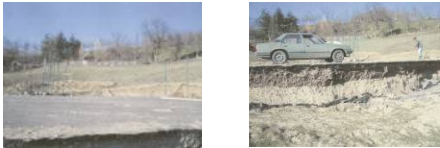
Slika 6. Prirodni nagib padine i njeno oštećenje Figure 6 The natural inclination of the slope and its damage
